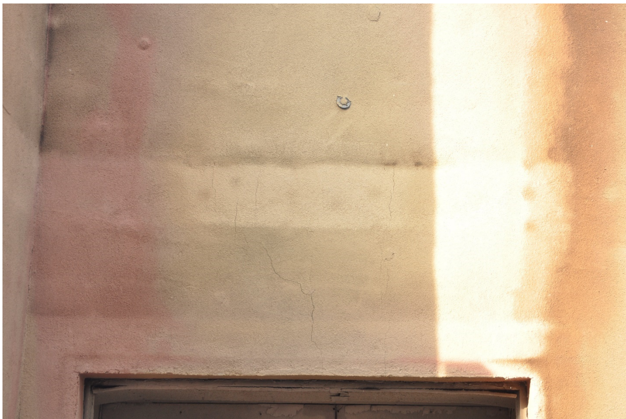
Figure 3.17: Visible cracks and fasteners in external coat
