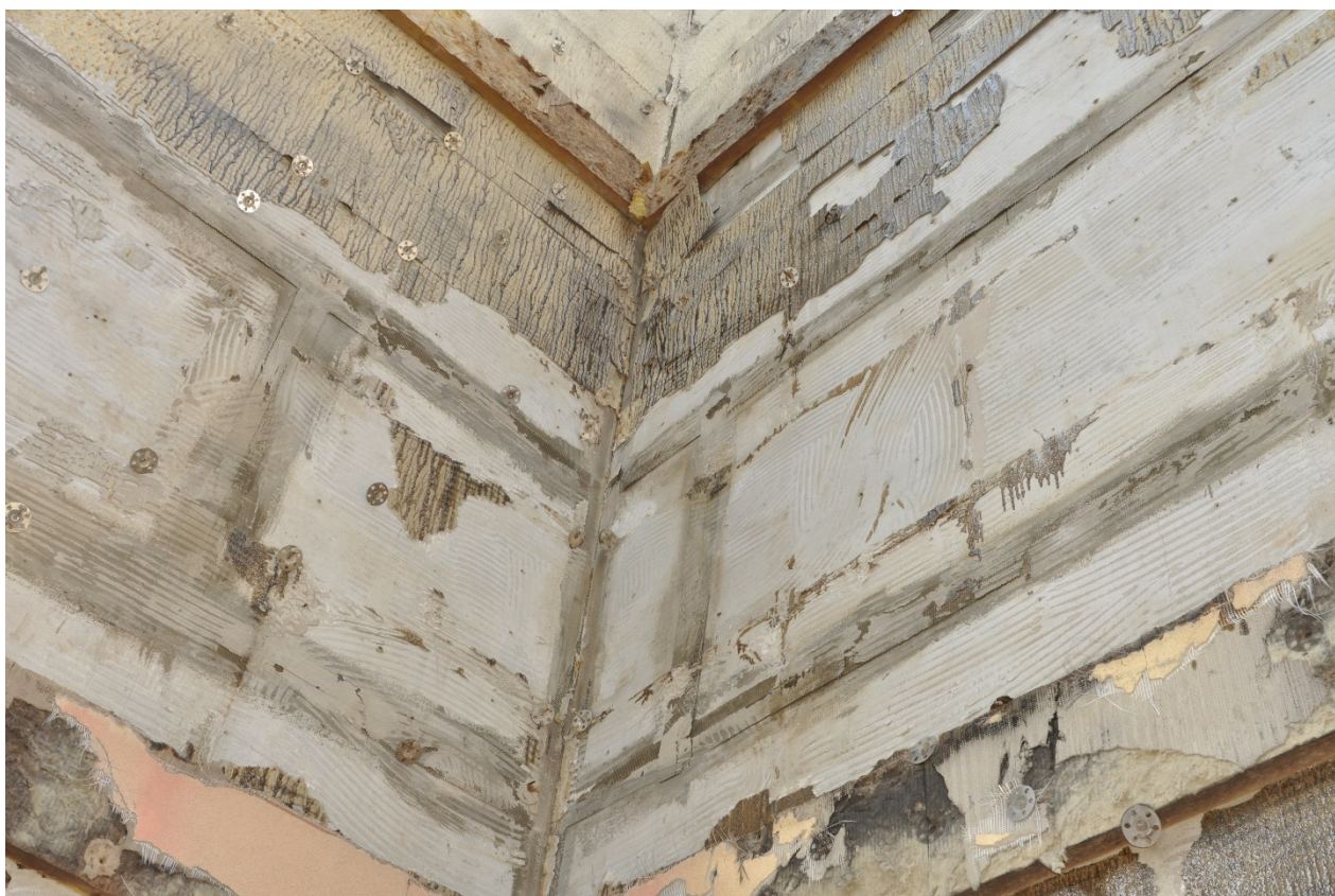
Figure 4.3: Condition of the board layer between the fire breaks
