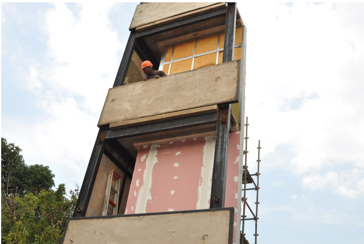
Internal boards fixed to the frame and plaster on joints and fixings
