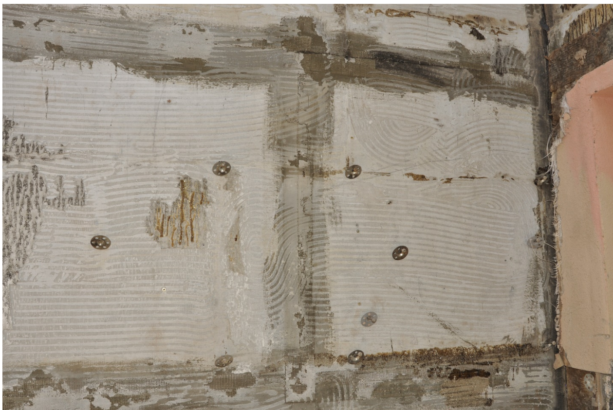
Figure 4.2: Condition of the board layer on the Wing Wall
